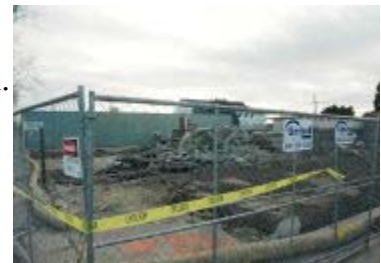
Auto California, formerly the San Pablo Florist and Nursery building, located at 1806 San Pablo Ave. as it appeared before and after its demolition last week.
